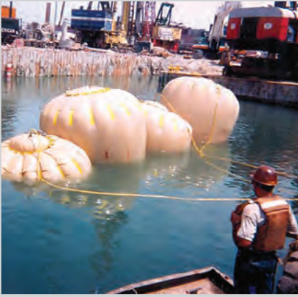
Professional lift bags used to lift a 100 ton concrete abutment during the Big Dig tunnel construction in Boston.
